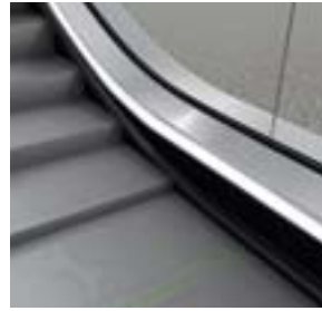
Continuous fiber optic skirt lighting
