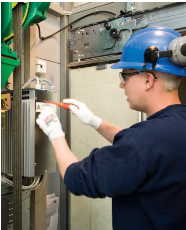
Our experienced modernization teams make sure the job is completed on time and on budget.
